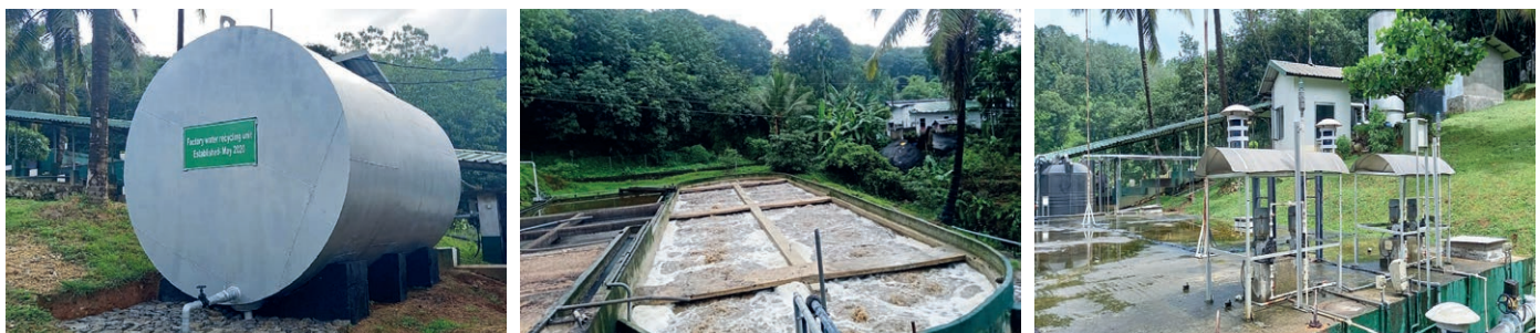
Processing water reutilisation unit and Effluent Treatment Plant at Dunedin Skim Rubber Factory
